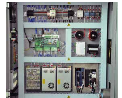
Conveniently designed industrialized wiring
